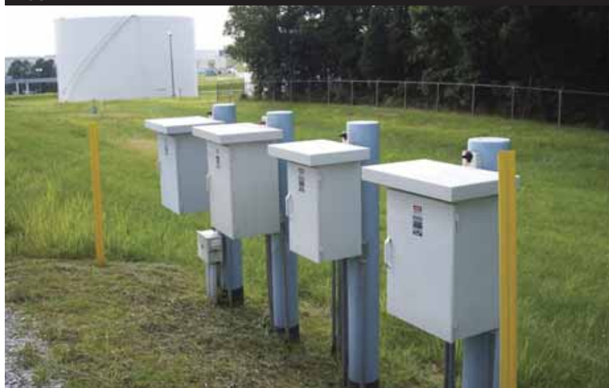
Rectifiers must be checked frequently to comply with regulations.
