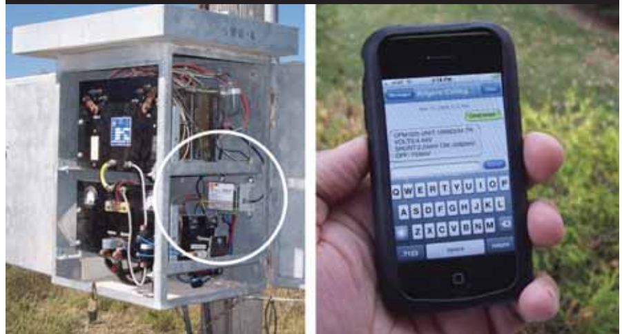
A remote monitoring unit (circled) installed at a rectifier, with cell phone communication.
