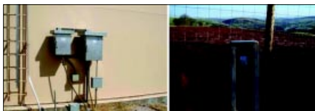
Figure 4: Monitoring (a) a T/R and (b): a CP point on a new LNG pipeline
